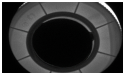
Valve with shifted inner lining
